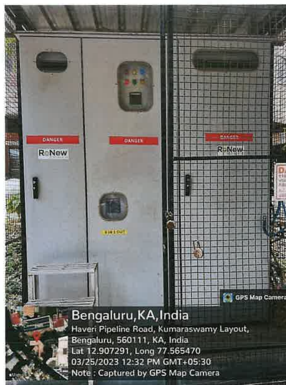
SOLAR ENERGY WHEELING METER BOARDS
