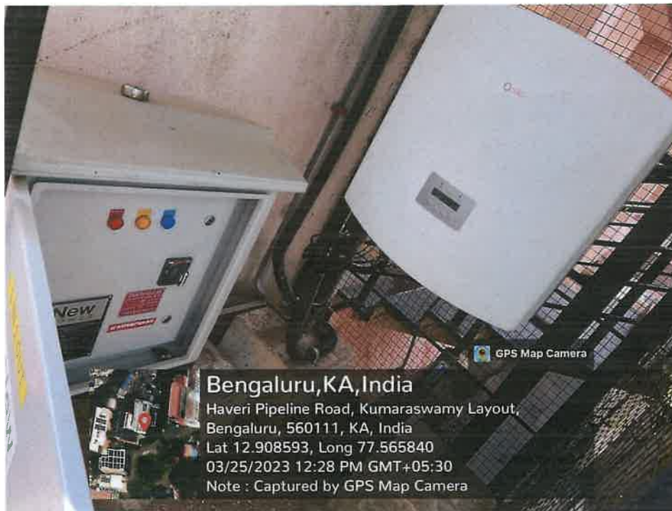
EQUIPMENT FOR WHEELING OF SOLAR ENERGY
