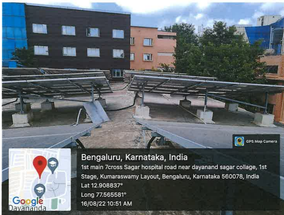
SOLAR ENERGY PANELS ON BUILDING ROOFTOP
