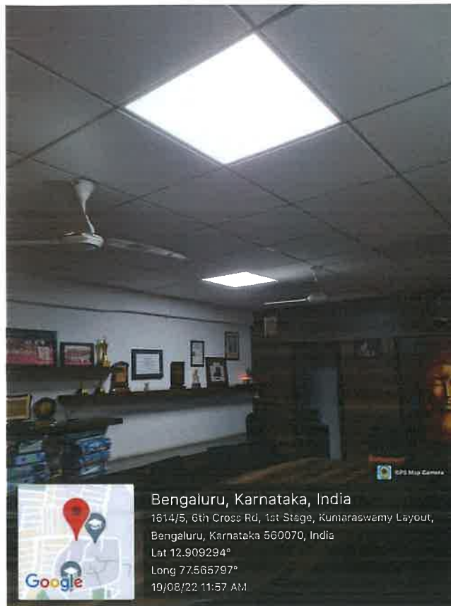
LED LIGHTS IN PRINCIPALS' OFFICE
