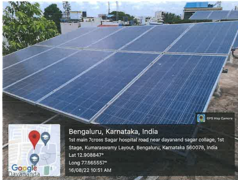
SOLAR ENERGY PANELS ON BUILDING ROOFTOP
